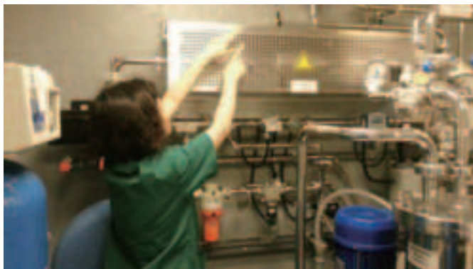
Figure 8: The stainless steel piping to carry the purified water to dialysis machines
